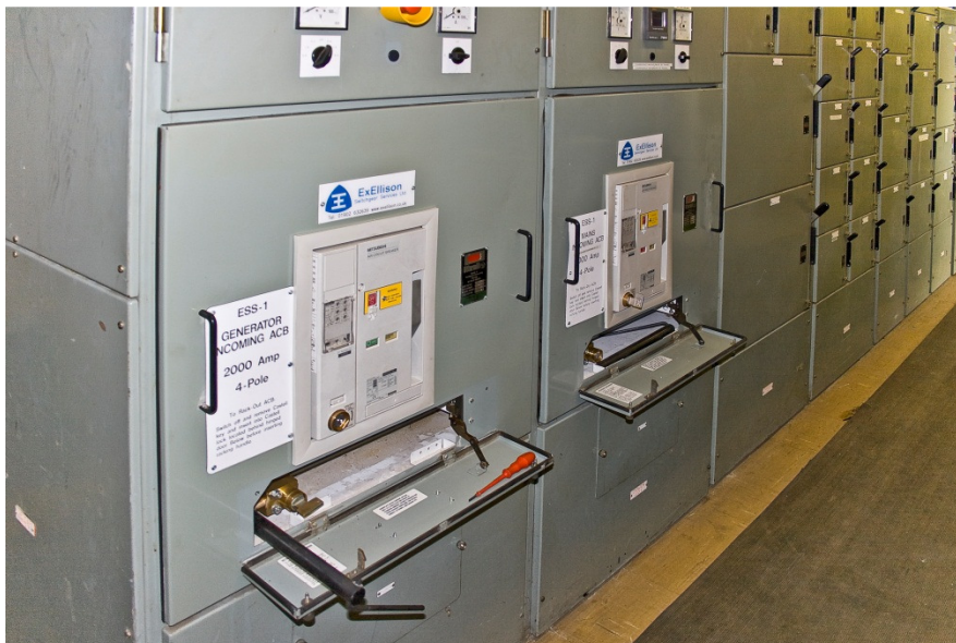
Upgraded Hospital switchboard
