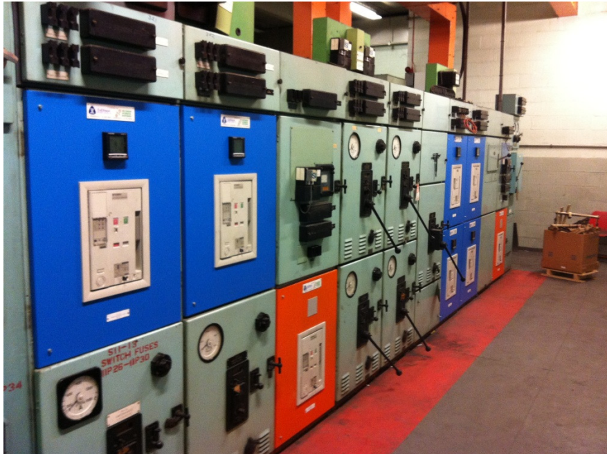
Partially retrofitted ACB switchboard at UK car plant.
